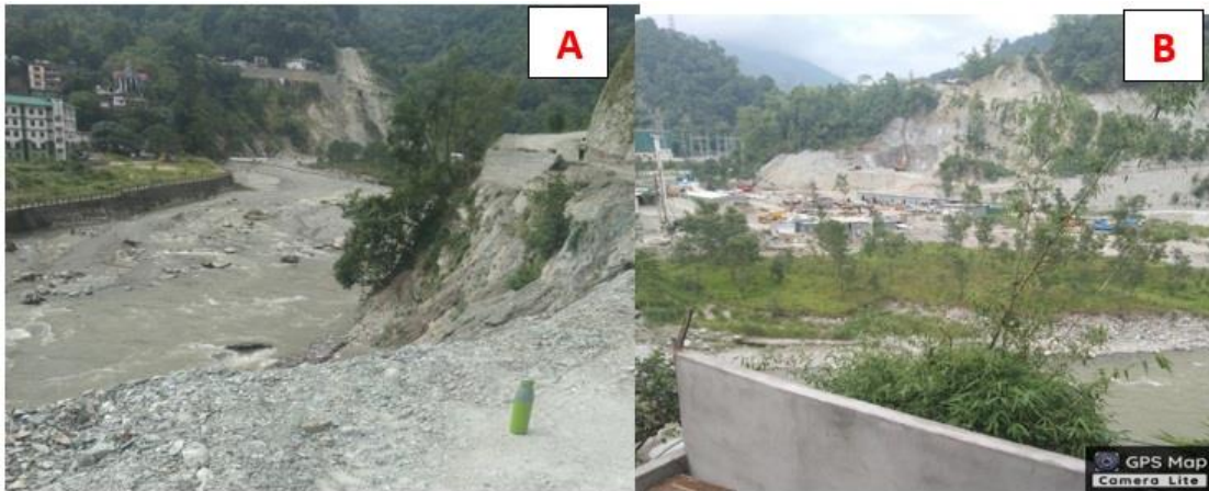
Figure 2.11. (A): Slope failure at the selected stretch of the Rangpochu due to landslides (27.13 N, 88.533 E) (B): Lateral Shift of lower terrace at the Rangpochu due to erosion ( 27.176 N, 88.532 °E)
