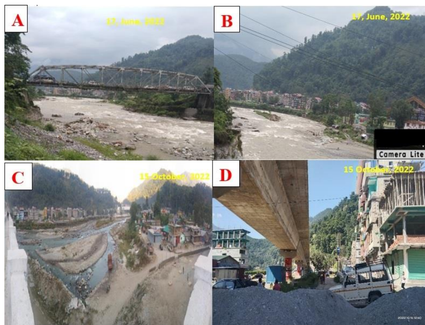
Figure 4.5. Built-up area in (Grid 23) along the Rangpochu (A): Rangpo bridge at the borderline of Sikkim and West Bengal which got cracked during heavy discharge flood in Oct 2021 (27.174 N, 88.53 E). (B): Built-up area downstream of Rangpo bridge (27.174 N, 88.529 E). (C & D): Built-up area at the confluence point of the Rangpochu and the Teesta (27.173 N, 88.524 E)
