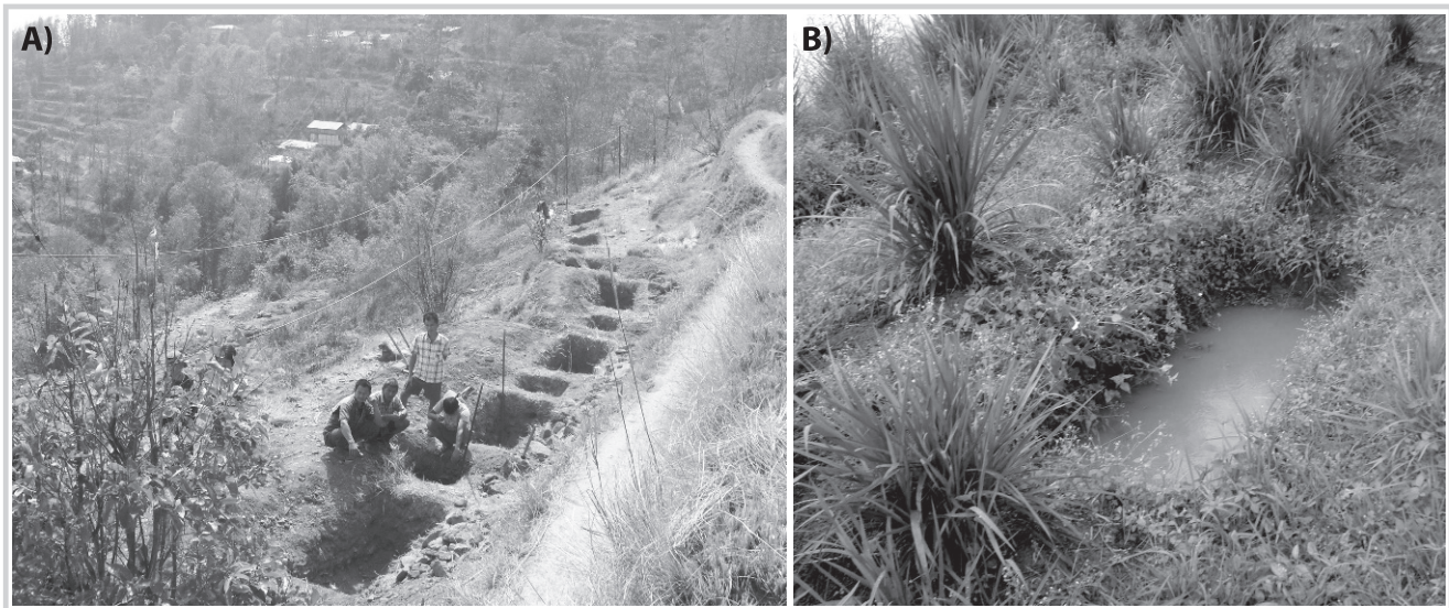
FIGURE 4 (A) Artificial recharge structures consisting of rows of rectangular staggered contour trenches (2 m × 0.8 m × 0.6 m) with square pits in between for mandarin orange horticulture plantations under construction in privately owned sloping lands in the recharge zone of Malagiri Dhara, Lungchok Kamarey Gram Panchayat, South Sikkim (May 2010) (Photo by Suren Mohra); (B) surface runoff trapped in the trenches assisting in artificial groundwater recharge along with fodder plantation in the recharge zone of Dokung Dhara, Takuthang Gram Panchayat, Kaluk block, West Sikkim (August 2010). (Photo by Pem Norbu Sherpa)
