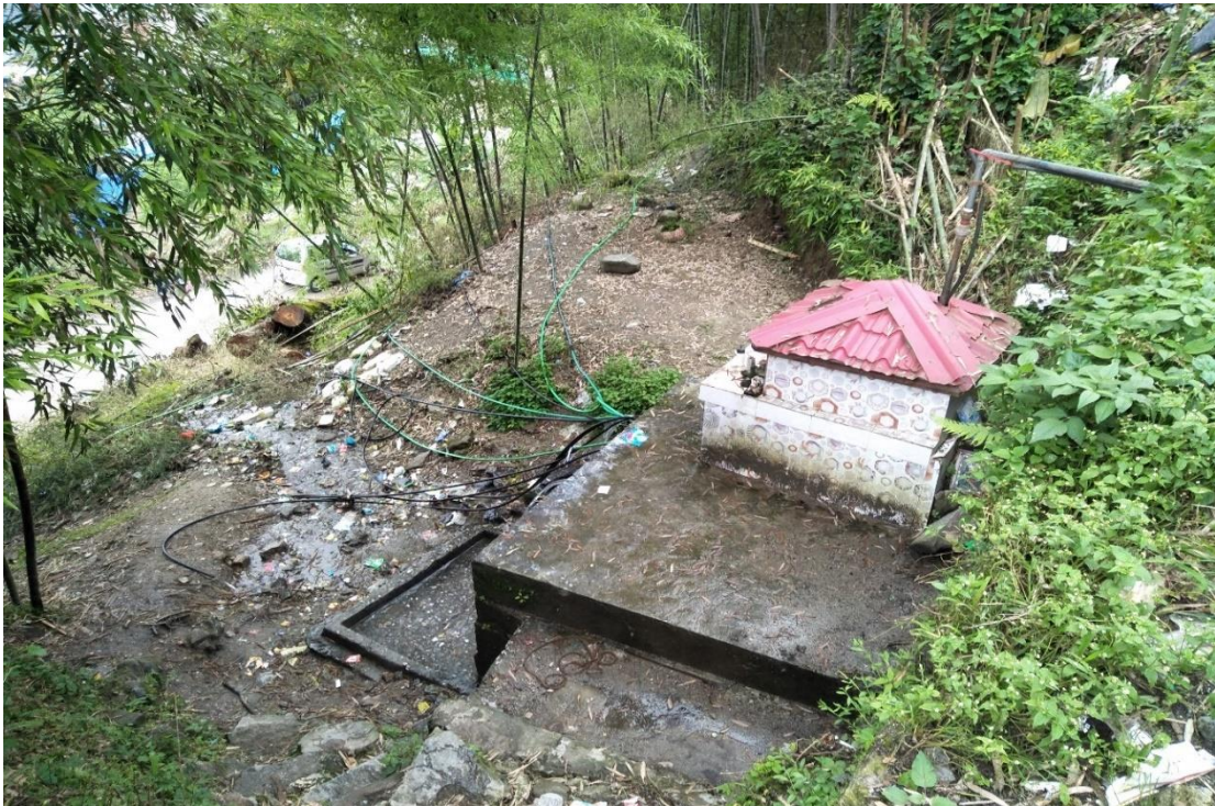
Figure 5.4: Privately Managed Water Connection and Reservoir
