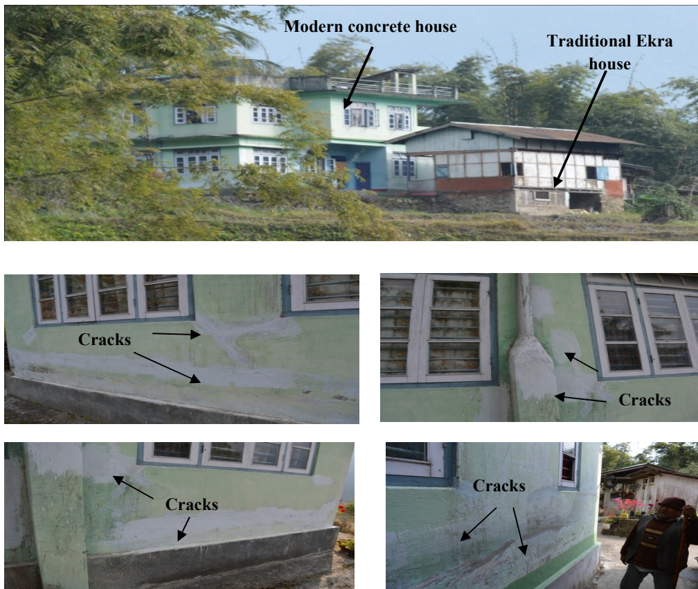
Plate IV.13: Impact of 18 th September, 2011 Earthquake on modern building structure in Sirwani village, East Sikkim
