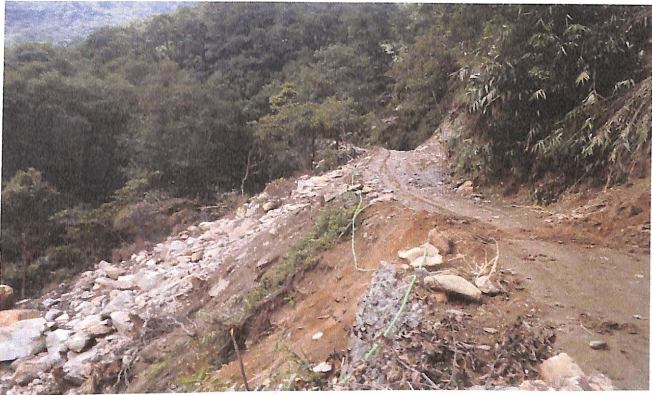
PLATE 7: Poor road connectivity due to Landslides
