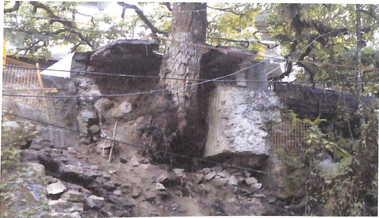
PLATE 11: House vulnerable due to slides and built under more active zone
