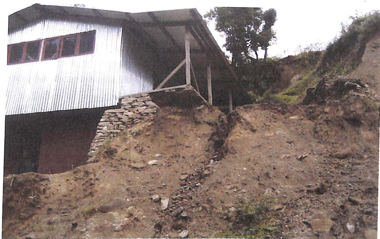
PLATE 12: House Knocked-Out by Landslide
